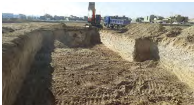
Preparation of the building site of the SFMC by the Iraqi general contracting party.
