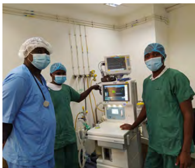
Joint work by experts from La Chaîne de l'Espoir and Malian biomedical technicians on the installation of a Dräger ATLAN 300 anesthesia apparatus at l'Hôpital du Mali (November 2021)
